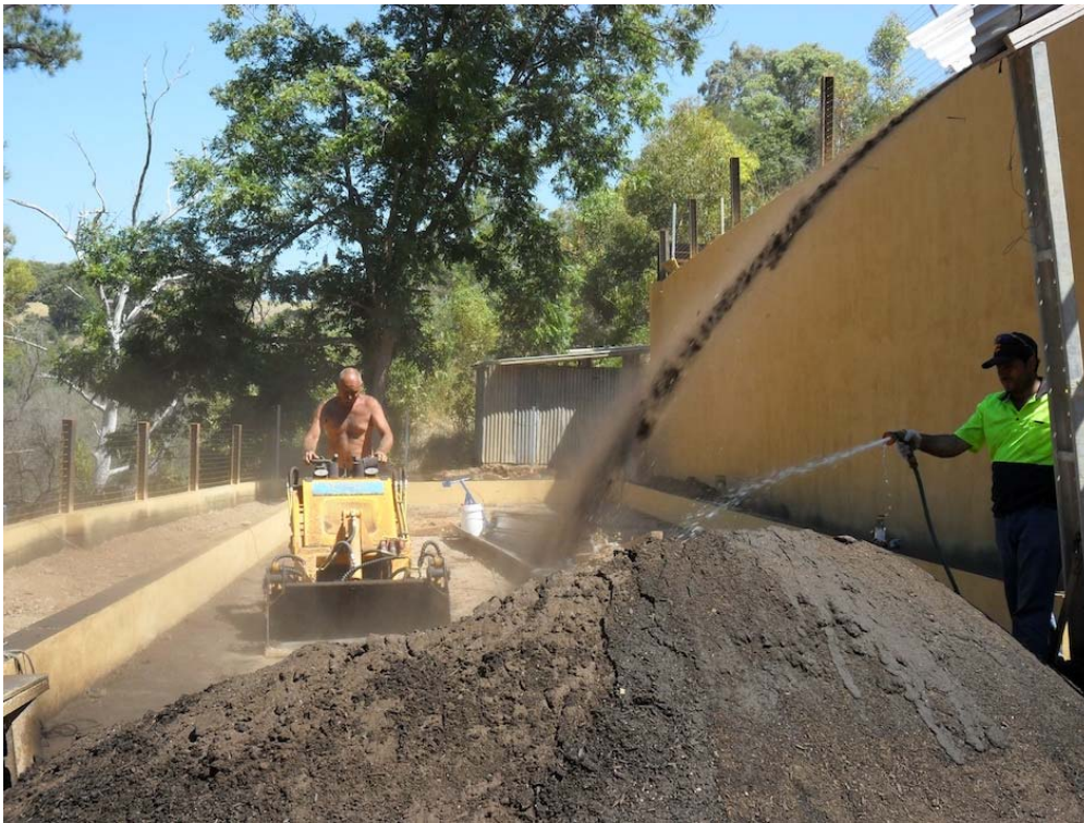
Middle level: Soil dropping out of the chute and being watered to reduce the dust. Roger is moving soil into the garden beds
